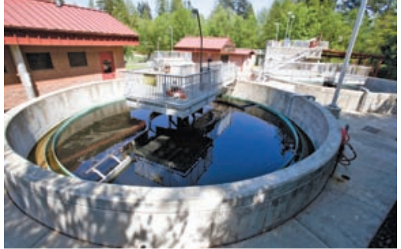
One of three final clarifiers at the Manchester plant.
